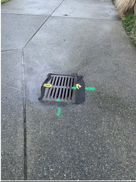
Catch Basin Point H driveway - West of 60 th Ave SE - Looking West
